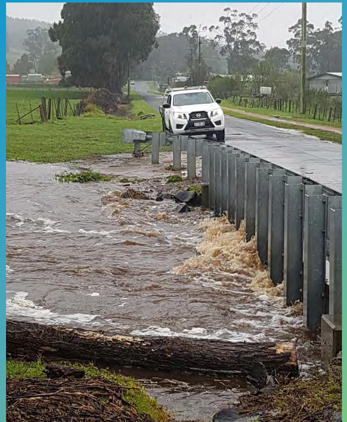
Dowbiggin Street, Railton during the October 2022 flooding event.
