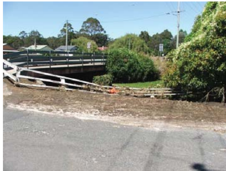
Foster St Bridge during and after the flood
