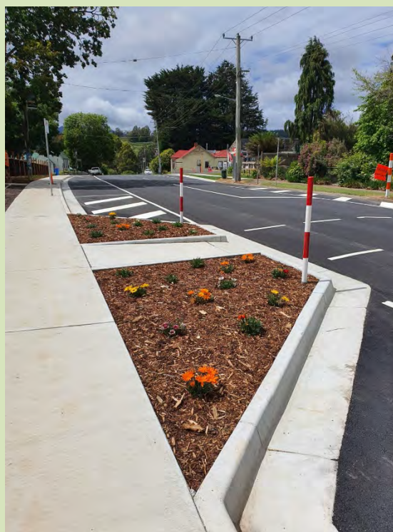
Wilmot's School Crossing was renewed as part of the Wilmot Main Street Upgrade Project.
